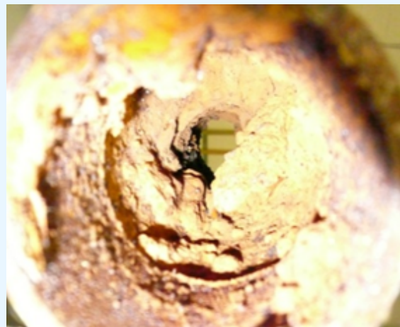
Limescale in a heating pipe, significant reduction in diameter.
