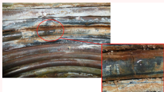
Limescale on surfaces lead to high temperature differences in the heat exchanger itself - thermal stress causes cracks with leaks.
