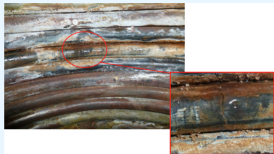
Limescale on surfaces lead to high temperature differences in the heat exchanger itself - thermal stress causes cracks with leaks.
